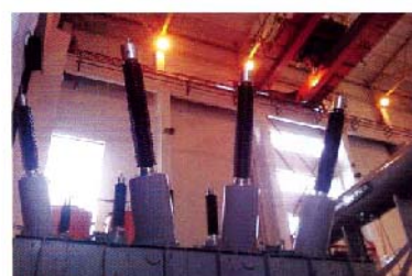
高中低压套管在沈阳随220kV变压器做突发短路试验 Bushings of 220kV transformer in sudden short circuit test
