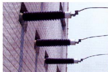
运行中的CRW-126/630-4型穿墙套管 Wall bushing in operation
